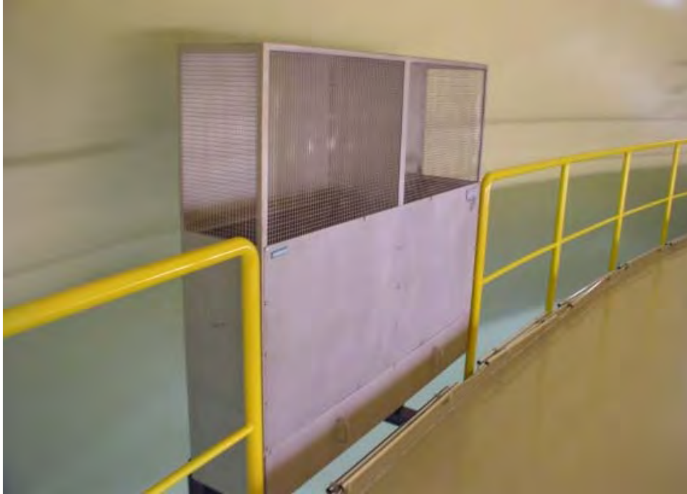
Figure 1: AREVA-design PAR inside a German PWR containment
