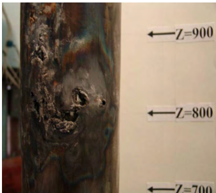
Fig. 7. View of the thermoinsulation shroud at the elevations of 700 – 900 mm.
